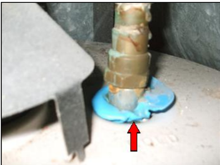
60. Carbon Monoxide/Heat spill over melted plastic
