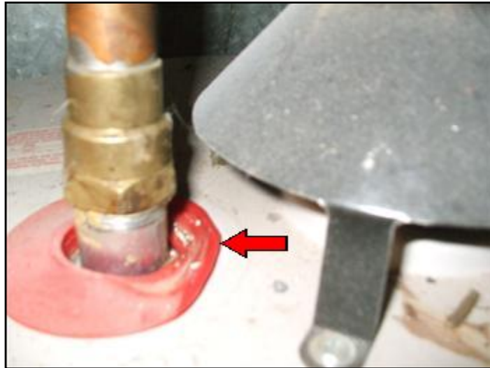
62. Carbon Monoxide/Heat spill over melted plastic
